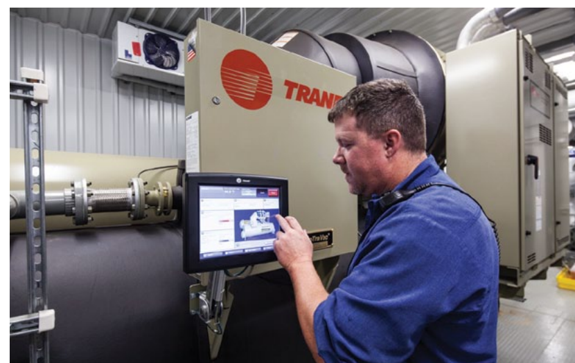
McCormick employee Charles DiStefano works with the new high-efficiency chiller.
